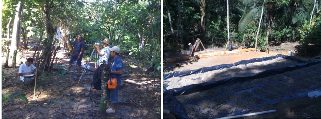
Figure 4. A) Personnel measuring levees and levels in the selected site. B) View of the three agriculture beds part of the IAAS system
