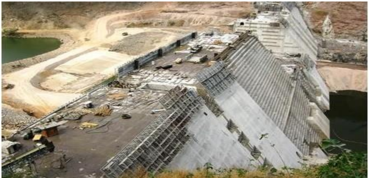
Plate R: A view of the late construction works at the Bui dam (Picture taken, November 2012)
